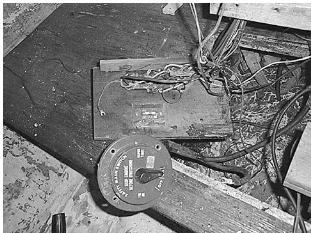
The electrical "system" I found on my MacGregor 222.
